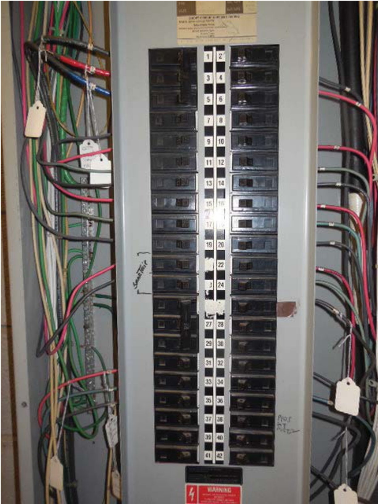
Picture 4: F11 Branch Ave. – Panel MES3 in Room C203
