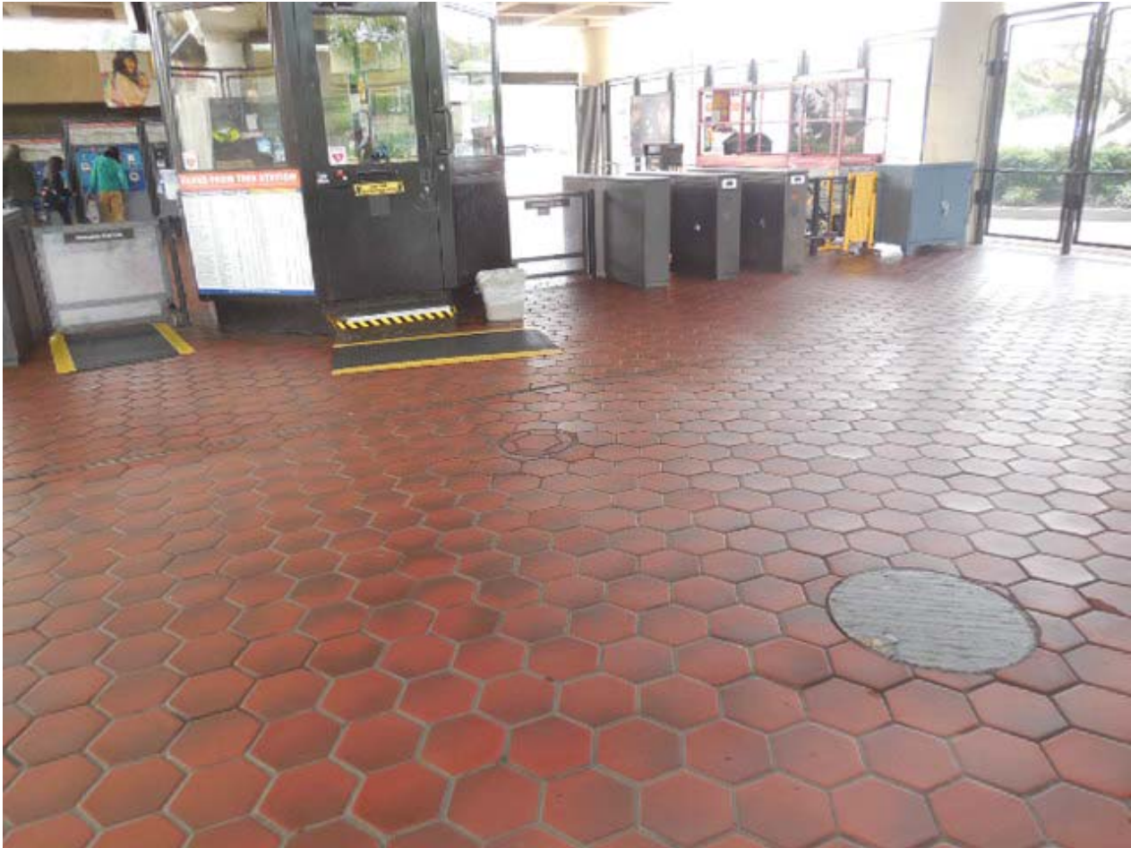
Picture 1: F09 Naylor – Handhole and manhole in mezzanine
