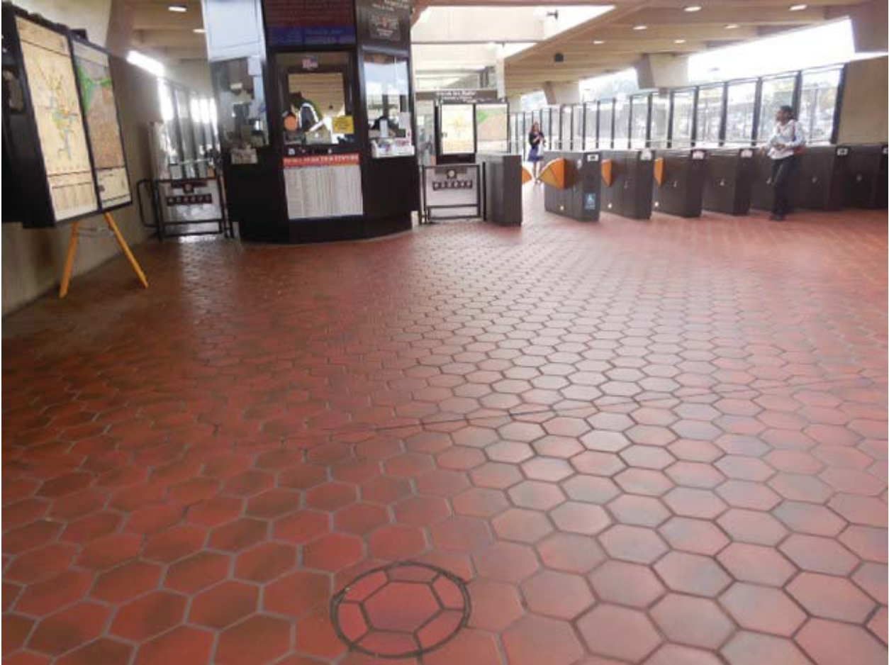
Picture 2: F11 Branch Ave. – Handhole in Mezzanine
