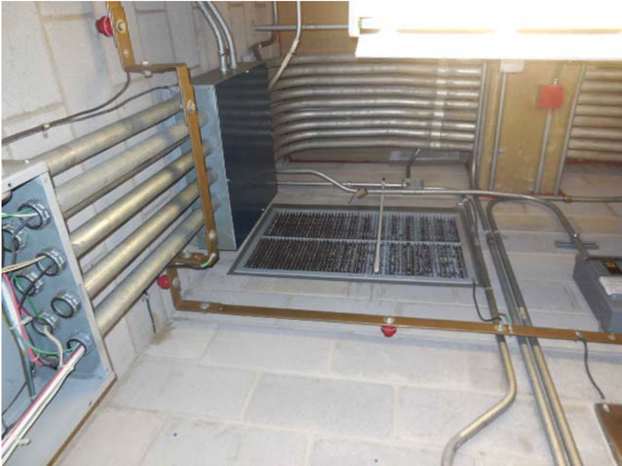
Picture 6: F11 Branch Ave. – Panel MES3 conduits to ceiling in Room C203
