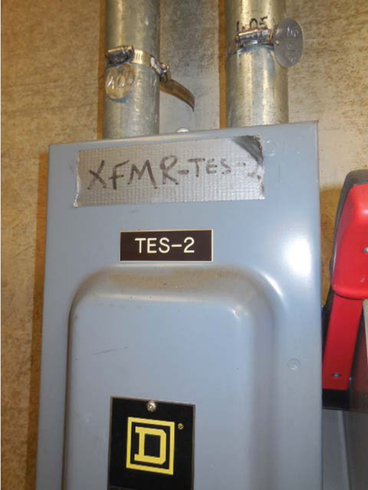
Picture 9: F11 Branch Ave. – Transformer disconnect switch TES-2 in Room C203
