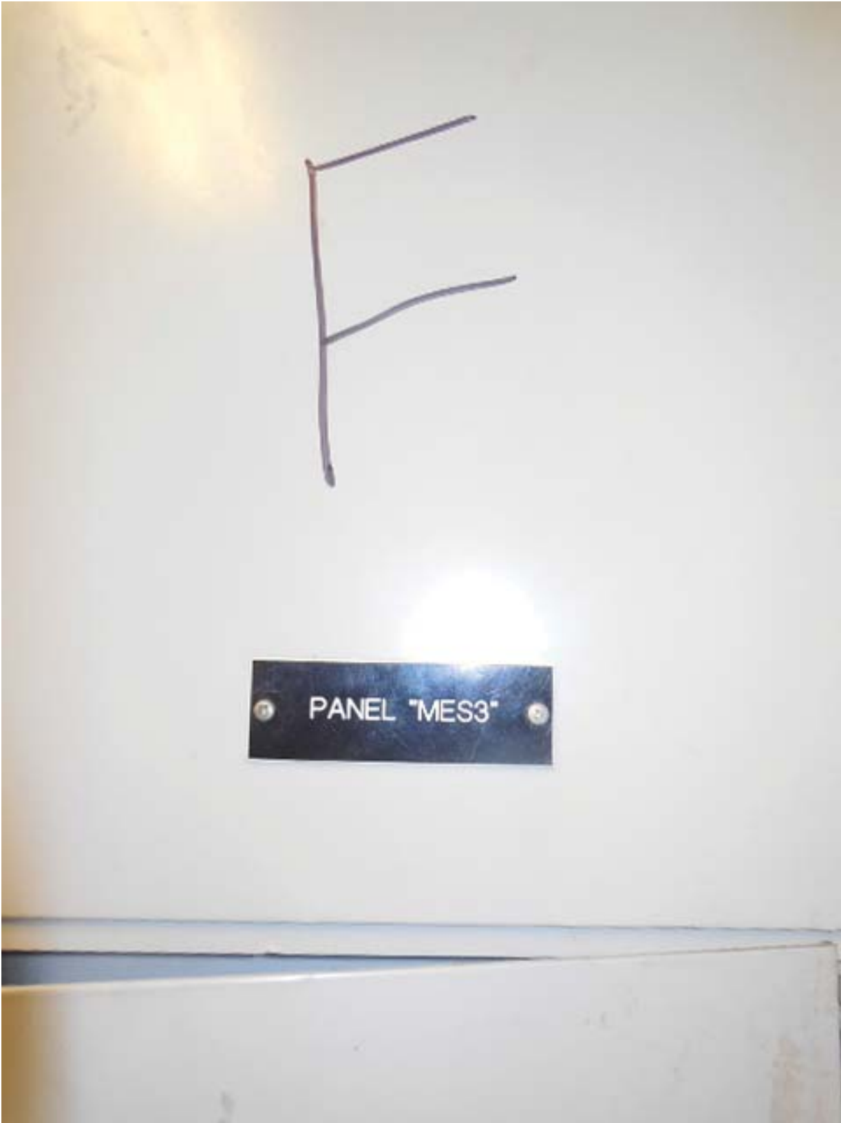
Picture 3: F11 Branch Ave. – Panel MES3 in Room C203
