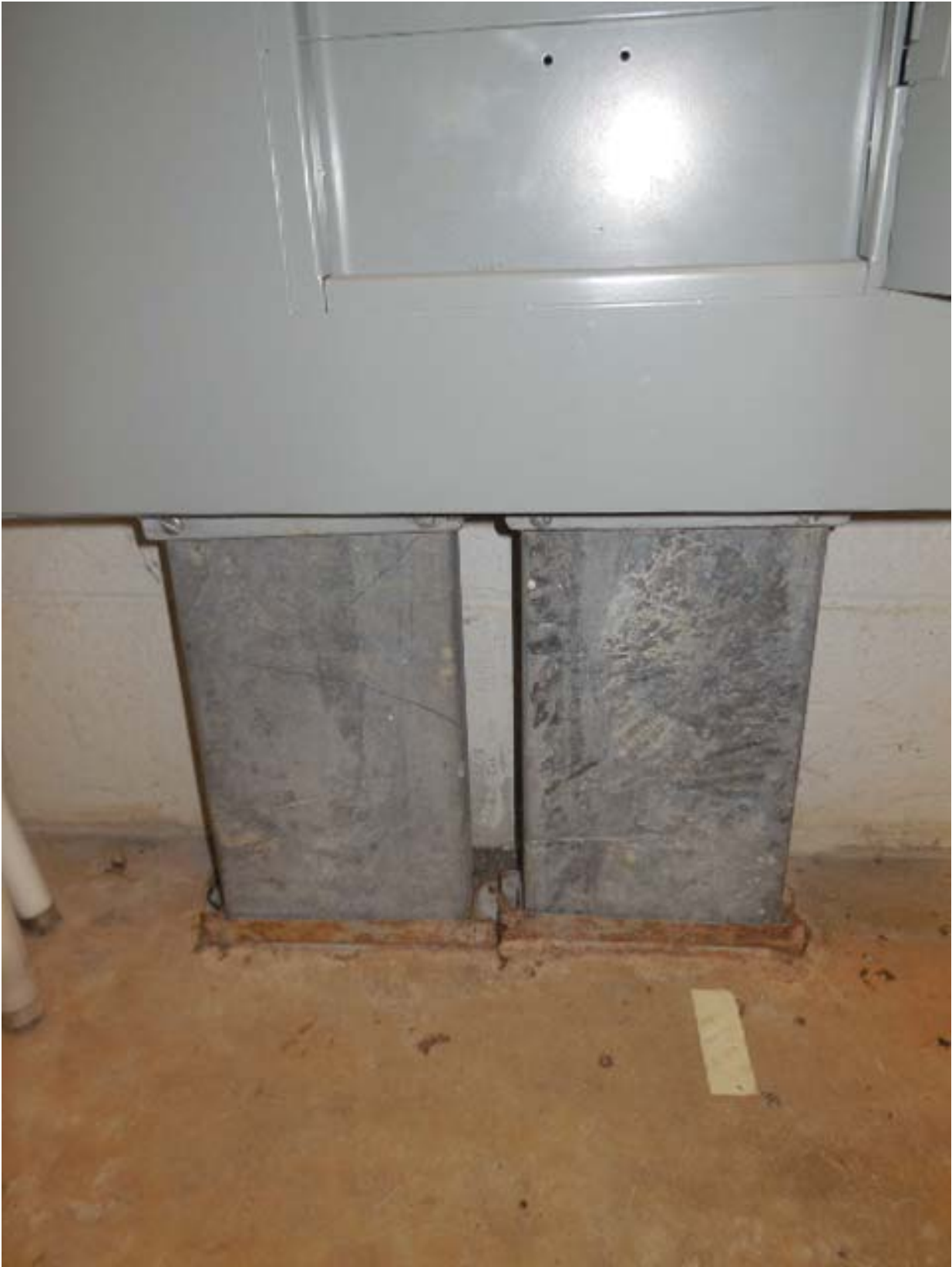
Picture 6: F09 Naylor – Bottom ducts of Panel MESS-2 in Room 126
