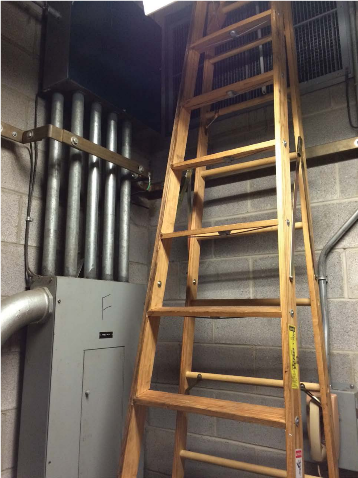
Picture 5: F11 Branch Ave. – Panel MES3 in Room C203
