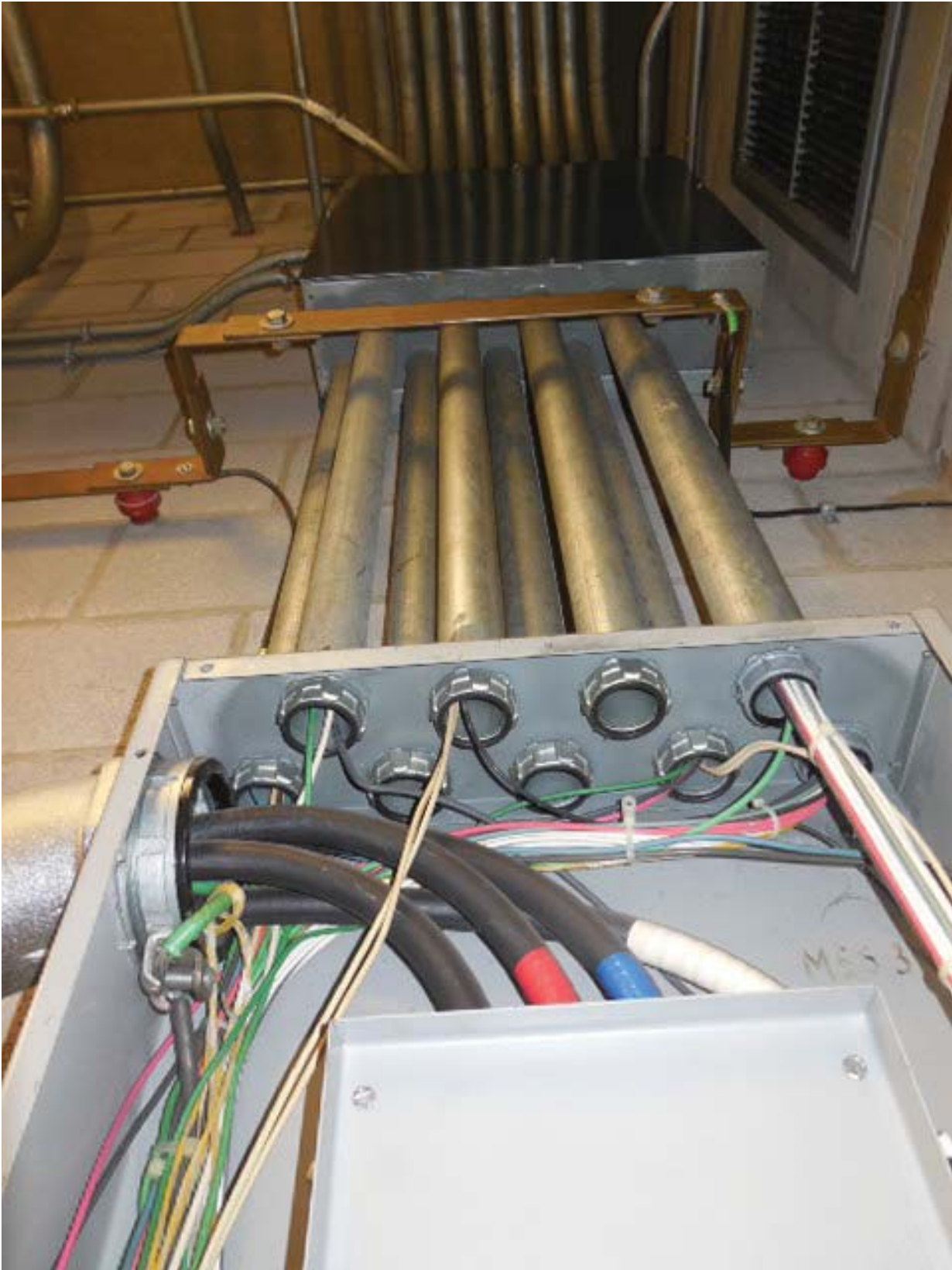
Picture 7: F11 Branch Ave. – Panel MES3 conduits to ceiling in Room C203
